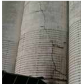
Pict. 4: Silo cell after fire
