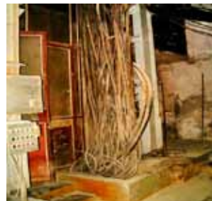
Pict. 8: Irregular cable management
