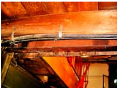
Pict. 7: Irregularly laid cables
